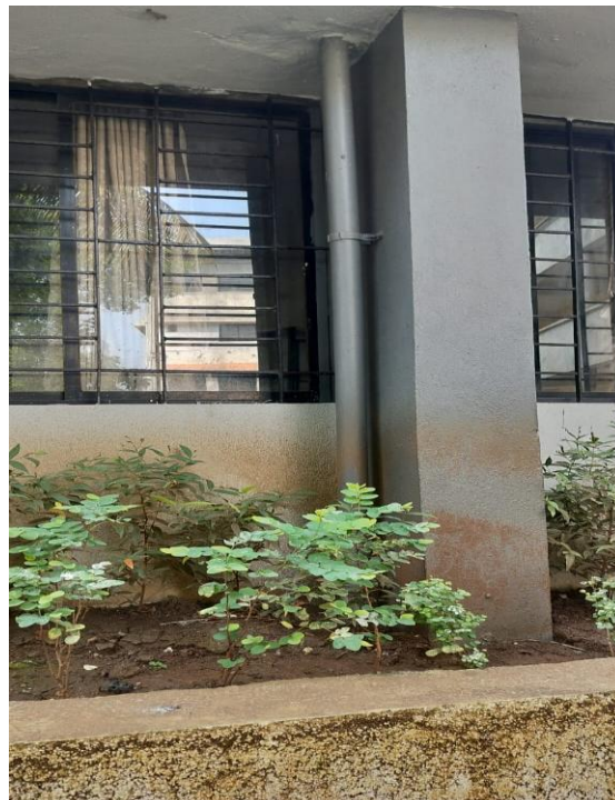
Rainwater collection pipe for Ground water recharging:
