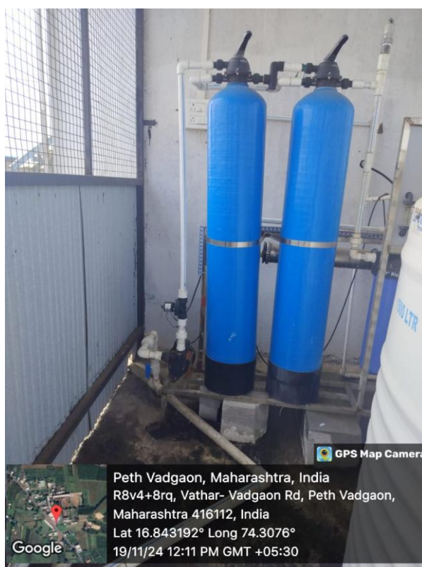
R.O water filter Unit
