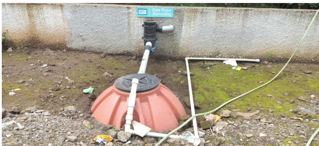
Advanced water filter unit
